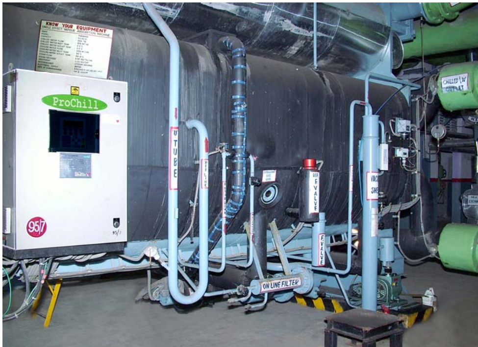
Vapour Absorption Machine ( Substitution of Energy )
