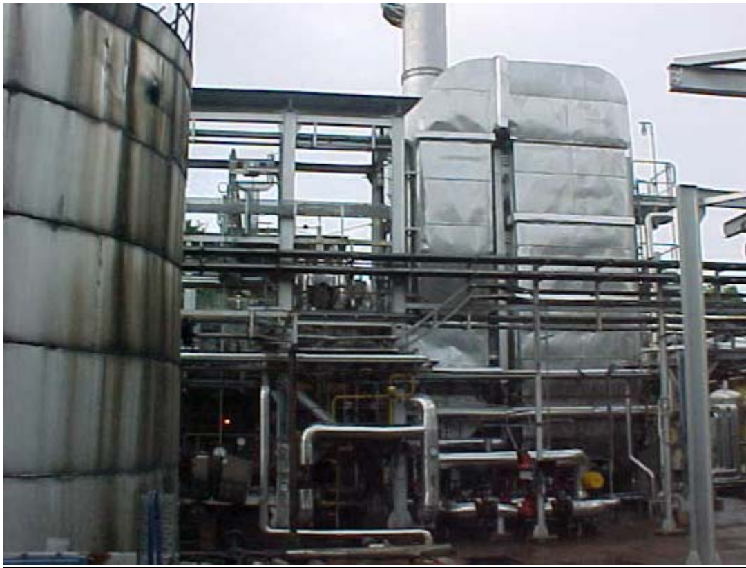
Photograph of '2 x 50 Tonnes Package Boilers'
