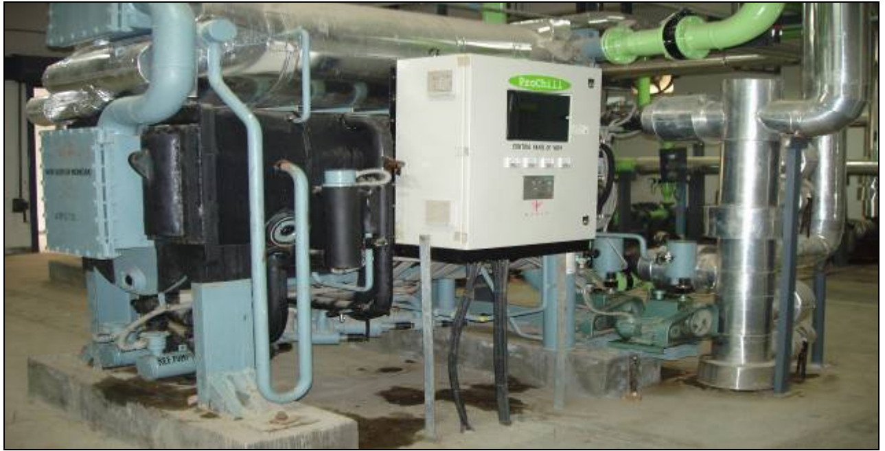
VAM (VAPOUR ABSORPTION MACHINE) INSTALLED AS AN ENERGY CONSERVATION MEASURE , POWER SAVED : 940 MW /YEAR
