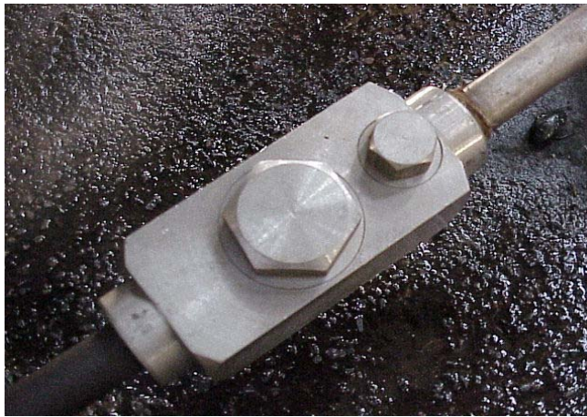
(view of new steam trap (low noise and Zero live steam loss))
