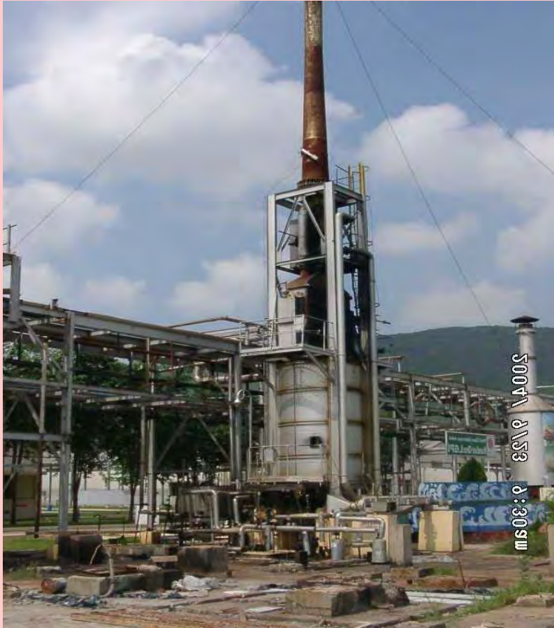
Old fired heater
