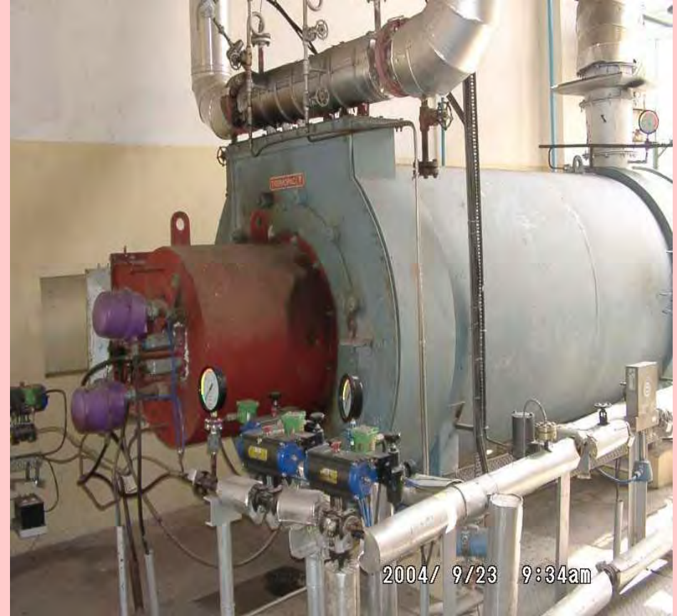
New fired heater
