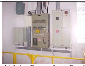
Lighting Energy Saver Panel for Slide Making Department
