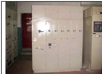
Main Lighting Energy Saver Panel
