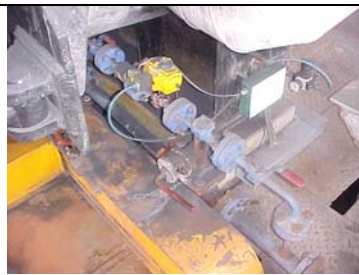
Automatic Blowdown System
