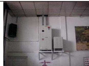
Lighting Energy Saver Panel for Canteen
