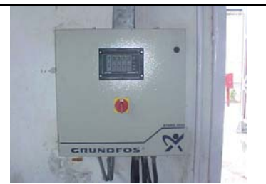
Control panel for interlocking Hi header pressure
