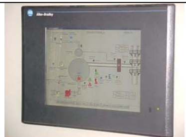
Online monitoring system
