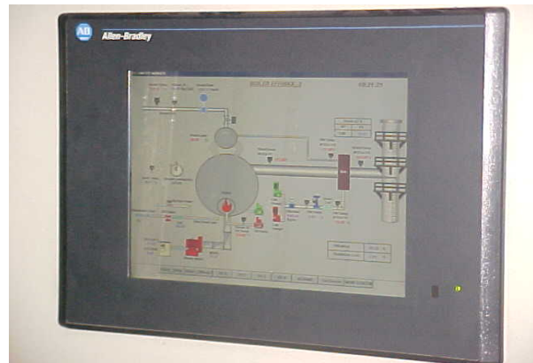
On line energy Monitoring system
