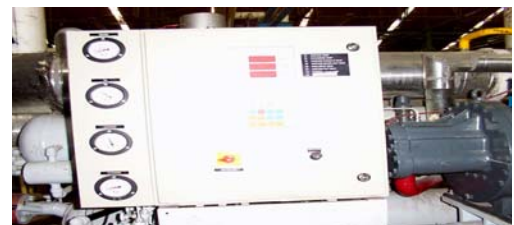
Reduction in load from 99 KW to 48 KW
