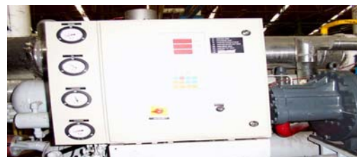
Reduction in load from 99 KW to 48 KW
