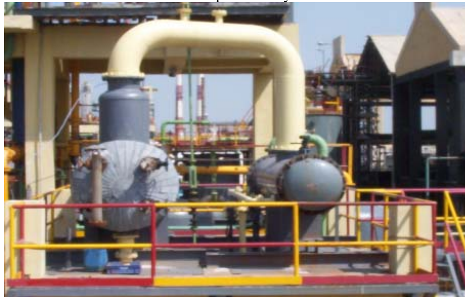
Flash Evaporation System
