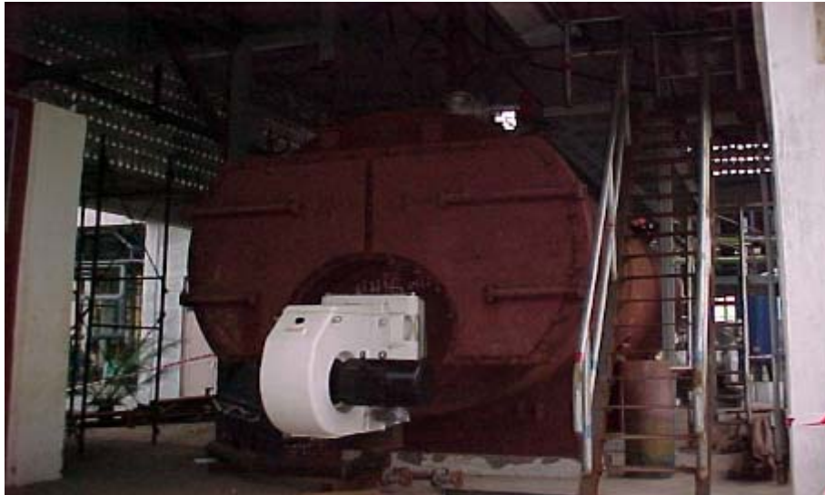
HYDROGEN FIRED BOILER
