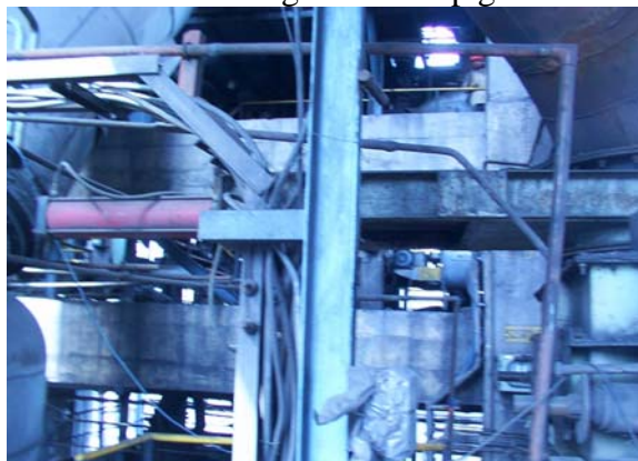
Slide gate for other circuit
