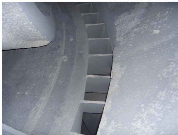
Raw mill modified dam ring
