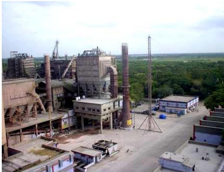
Electro Static Precipitator installed at clinker cooler
