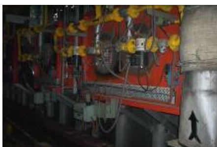
Coal Gas System at Preheater
