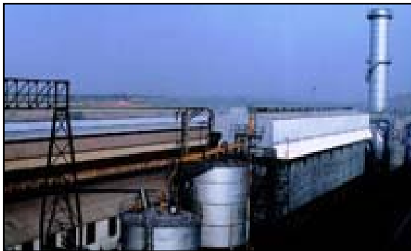
Fume treatment plant
