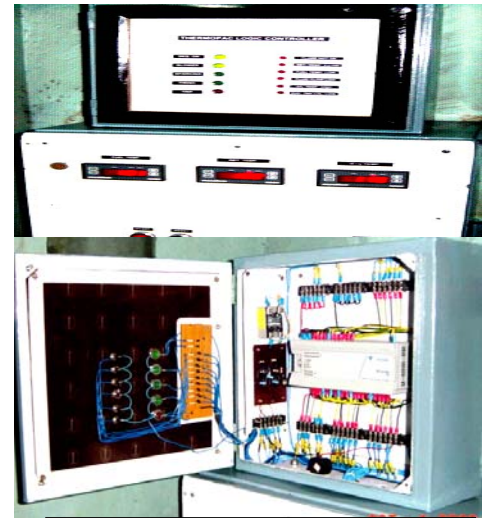
Thermopac control panel
