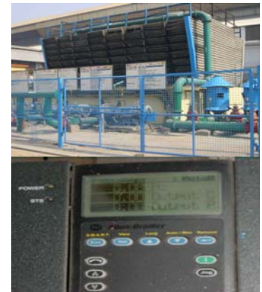
VFD in cooling tower
