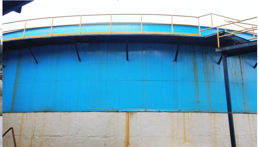
Clarifier without insulation
