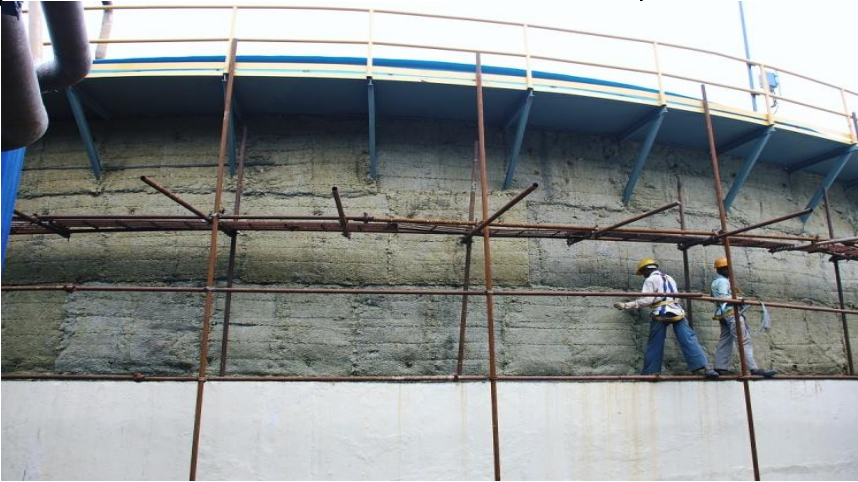
Clarifier with insulation and water seal.
