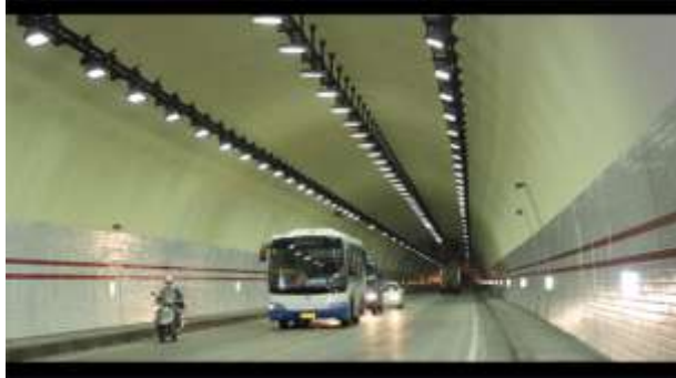
Underground Tunnel Lighting
