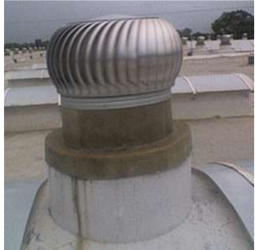
Use of Eco Friendly Ventilation System
