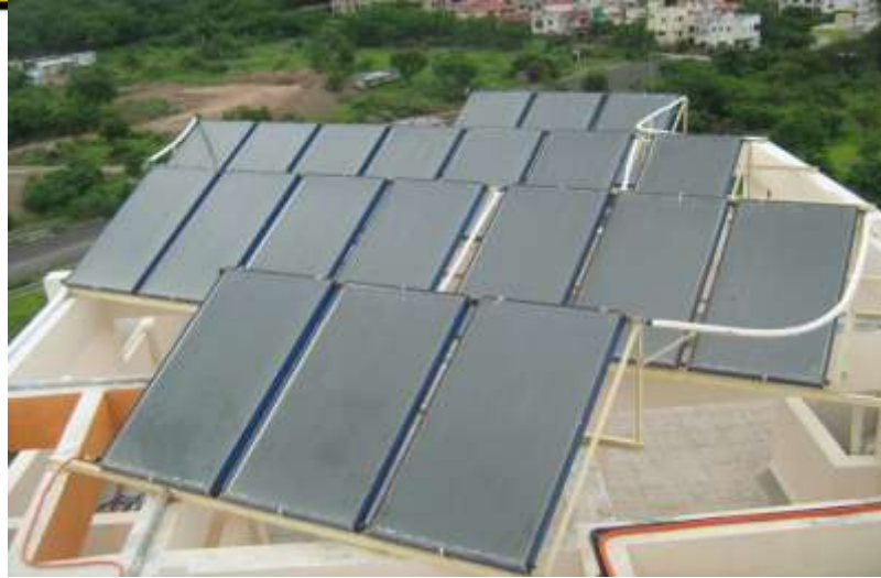
SOLAR WATER HEATING PANELS
