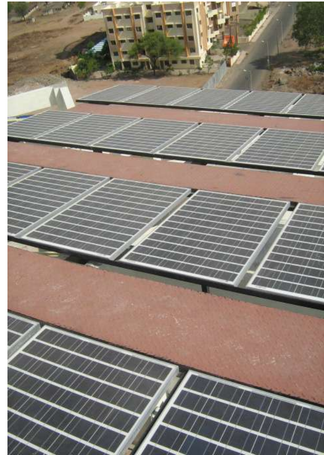
SOLAR PV-4.3 kw
