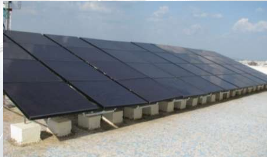
SOLAR PHOTO VOLTAIC PANELS ON THIRD FLOOR TERRACE
