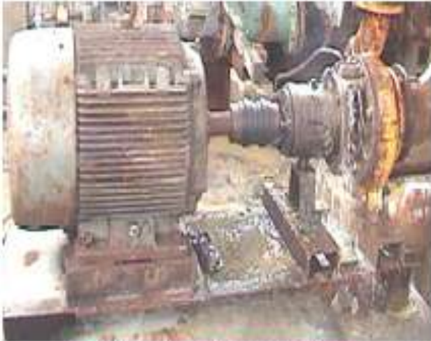
ETP PUMP, 55 KW MOTOR
