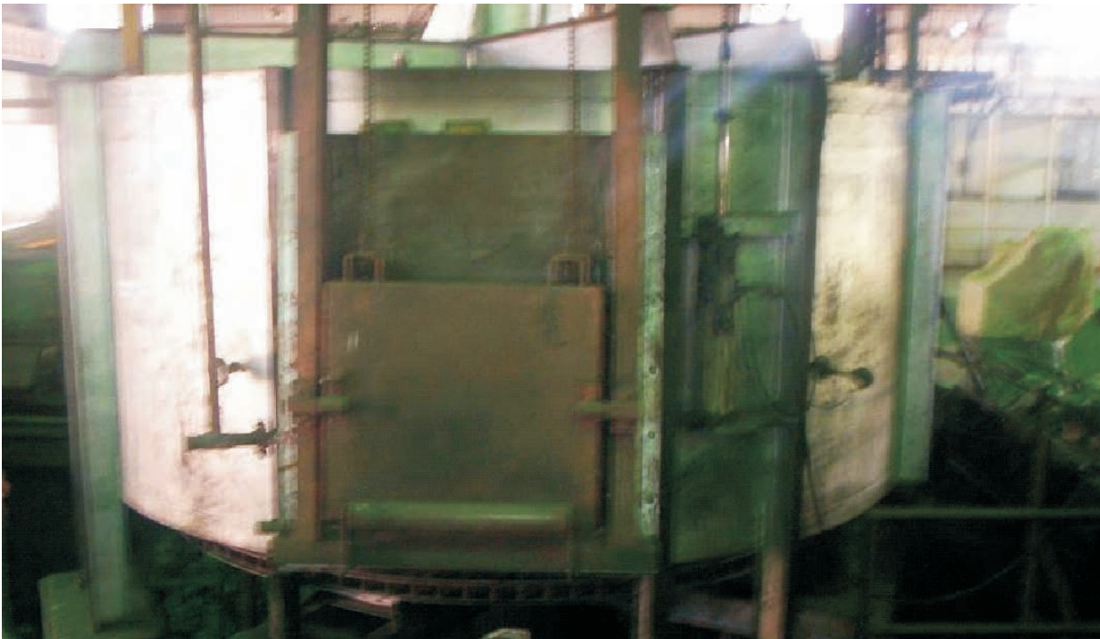
Rotary Furnace No.2 of 125 KW which is eliminated by C.G.C.F
