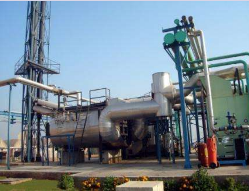
WHRB for 3 X 1 MW HSD fired engine
