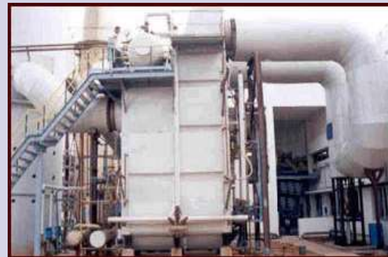
WHRB for 3.8 MW HFO fired engine
