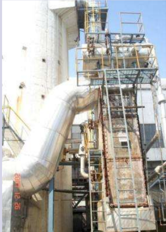
Hot waste gases from Glass Furnace
