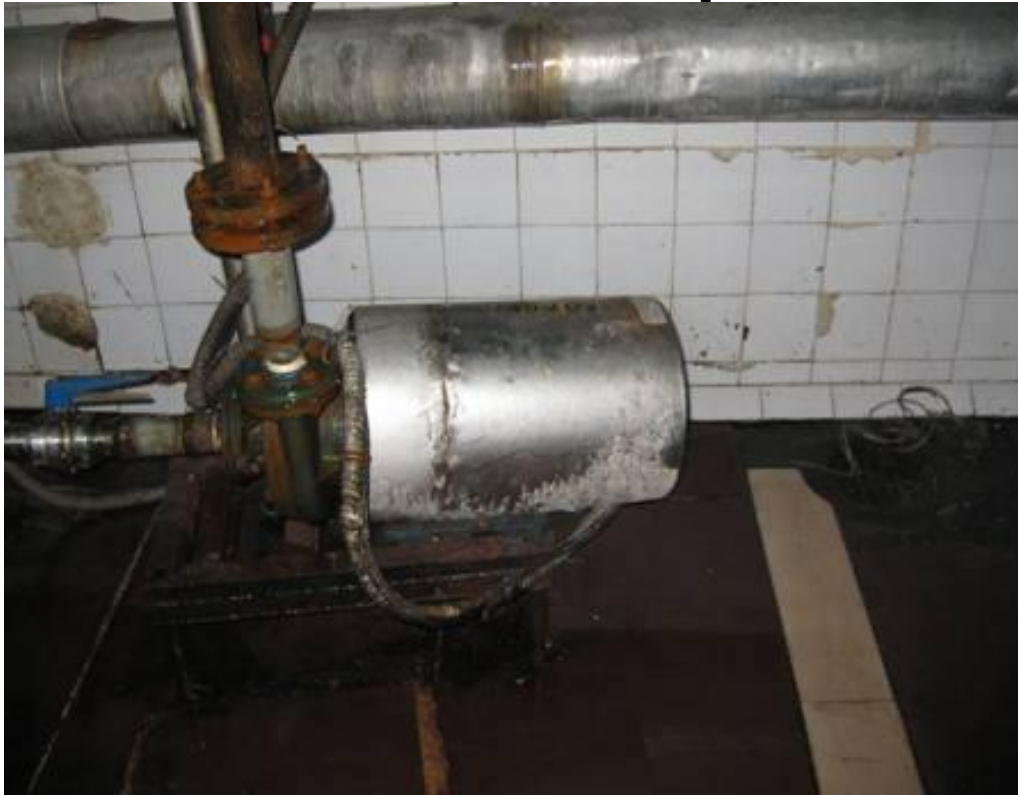
3 Hp Chilled Water Pump
