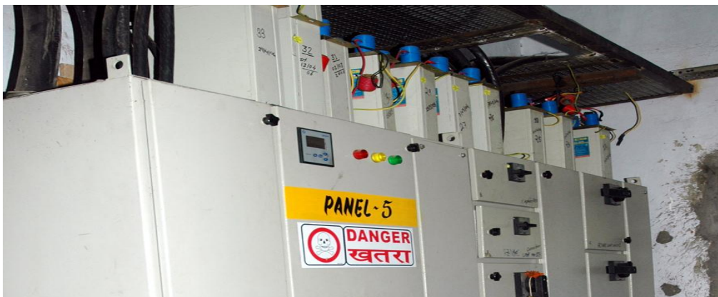
CAPACITOR BANK No. 1
