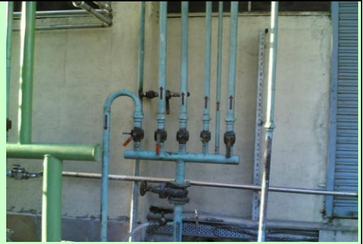
Old Water Distribution
