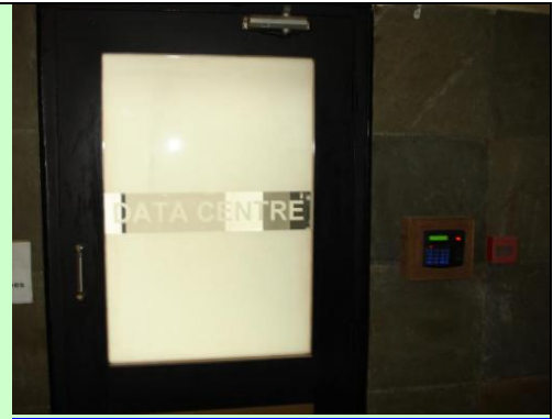
New Data centre
