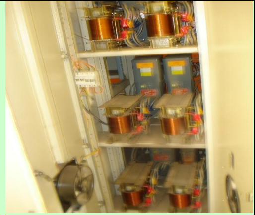
Harmonic control panel
