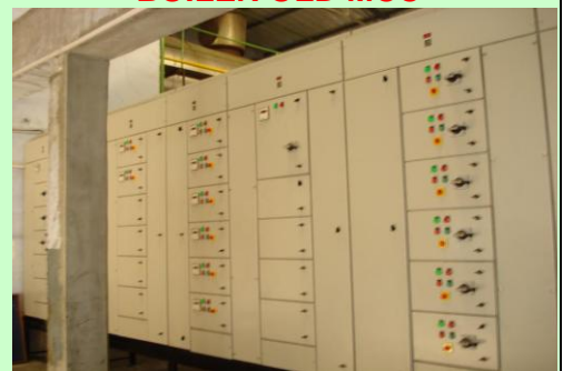
BOILER NEW MCC
