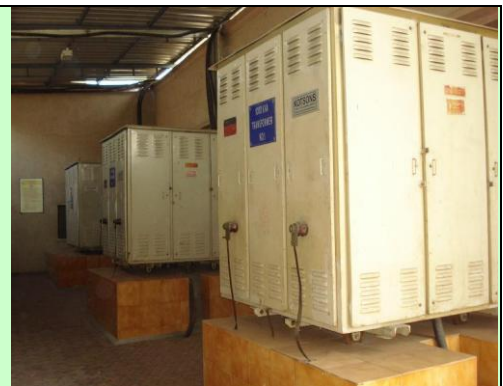
Loading on two transformer instead of three
