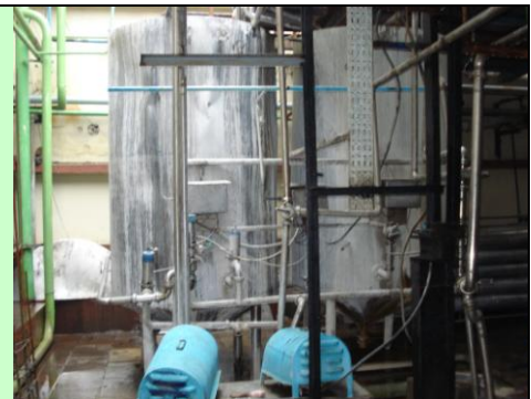
CIP with 3 hp Return Pump
