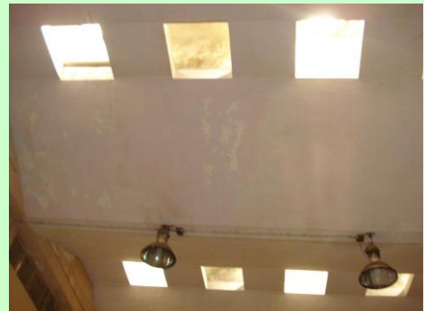
Ghee section with ventilation
