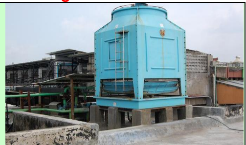
Air compressor cooling tower
