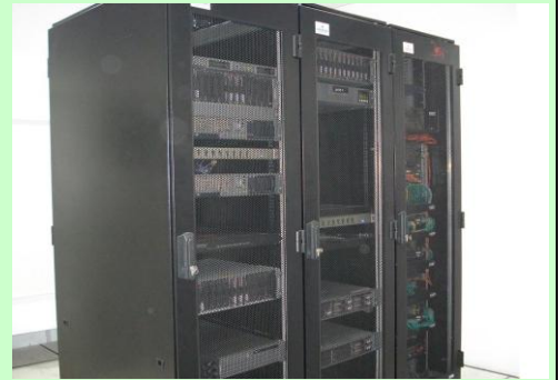
New Data centre
