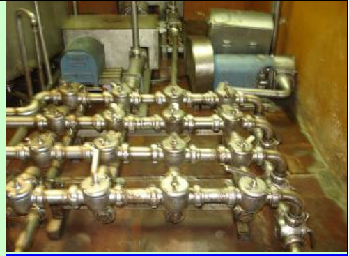
Cream transfer pump with VFD
