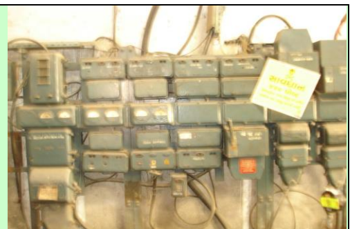
BOILER OLD MCC
