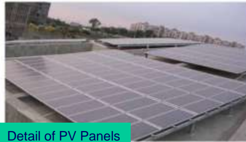
Detail of PV Panels
