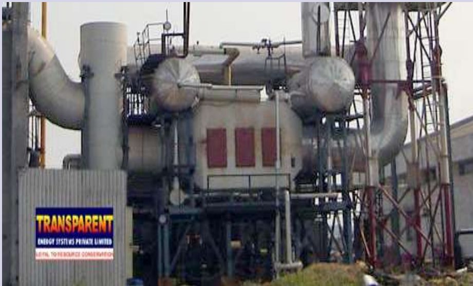
WHRB on 6.7 MW gas fired engine
