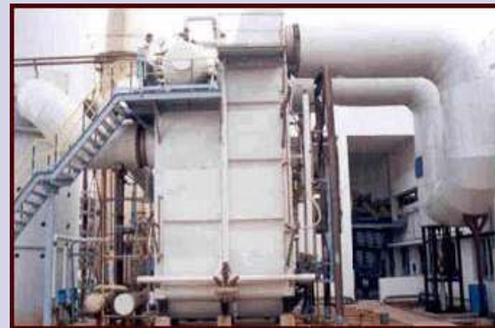
WHRB for 3.8 MW HFO fired engine
