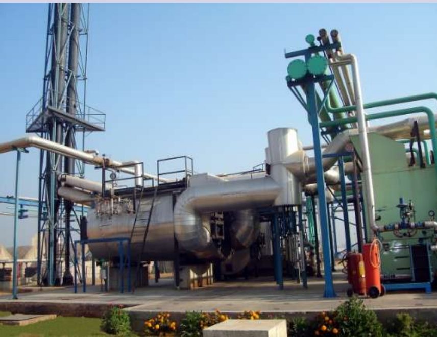
WHRB for 3 X 1 MW HSD fired engine
