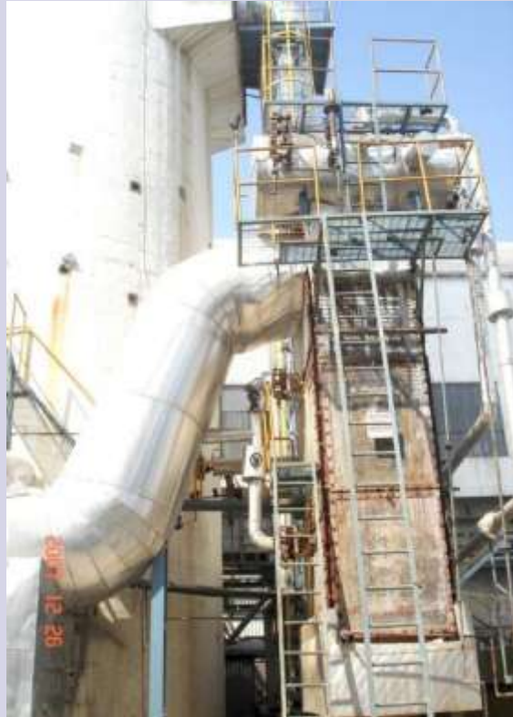
Hot waste gases from Glass Furnace
