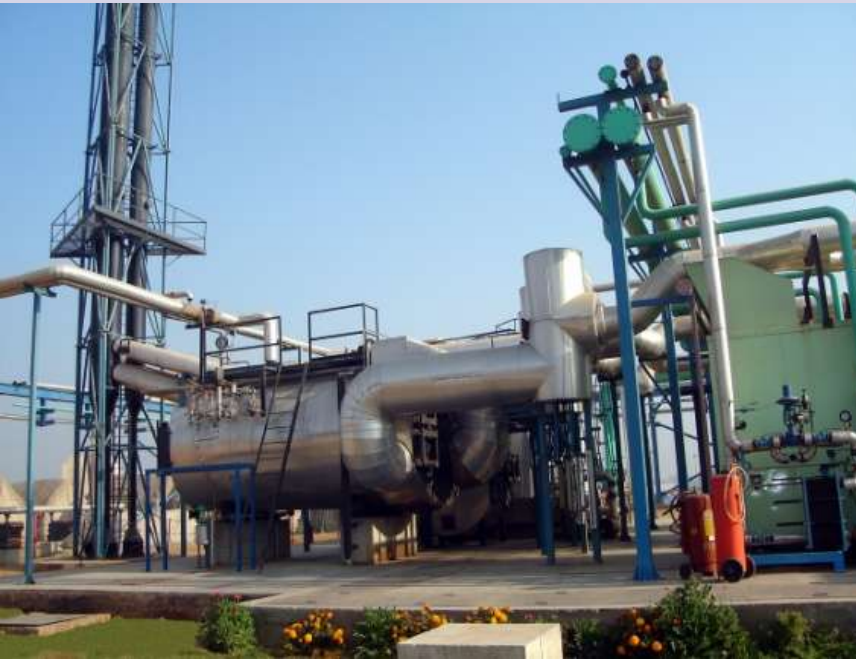
WHRB for 3 X 1 MW HSD fired engine
