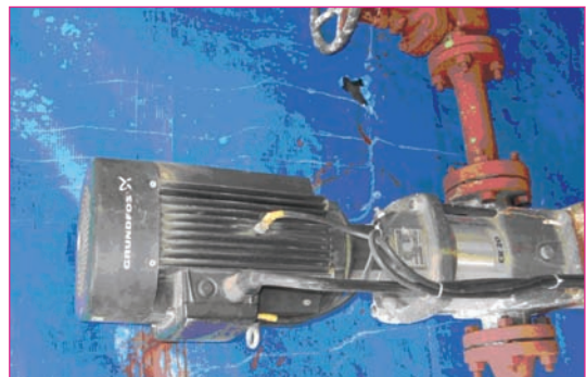
▲ New Small EE Grundfos Pump For Air Compressor
