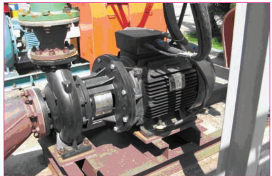
▲ New EE Grundfos Pump For AFC-2 Plant
