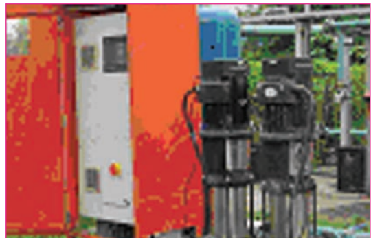
▲ Hydro-Booster system for filter water plant
