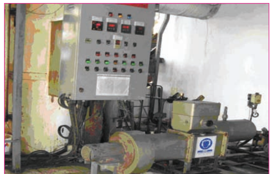
▲ Thermic Fluid Heater
