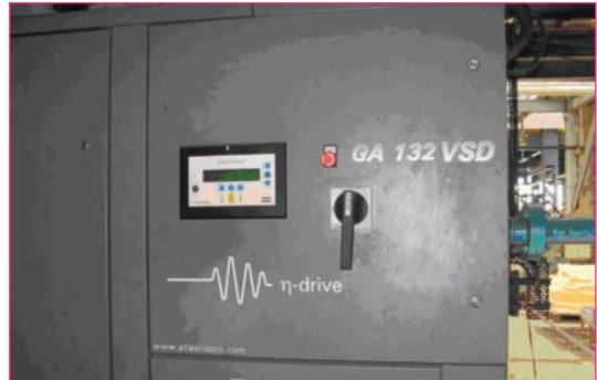
▲ New Air Compressor With VFD
