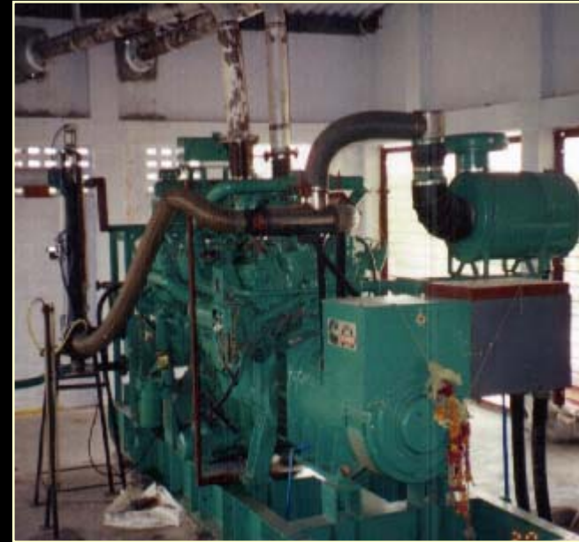
System Package : GAS-200
