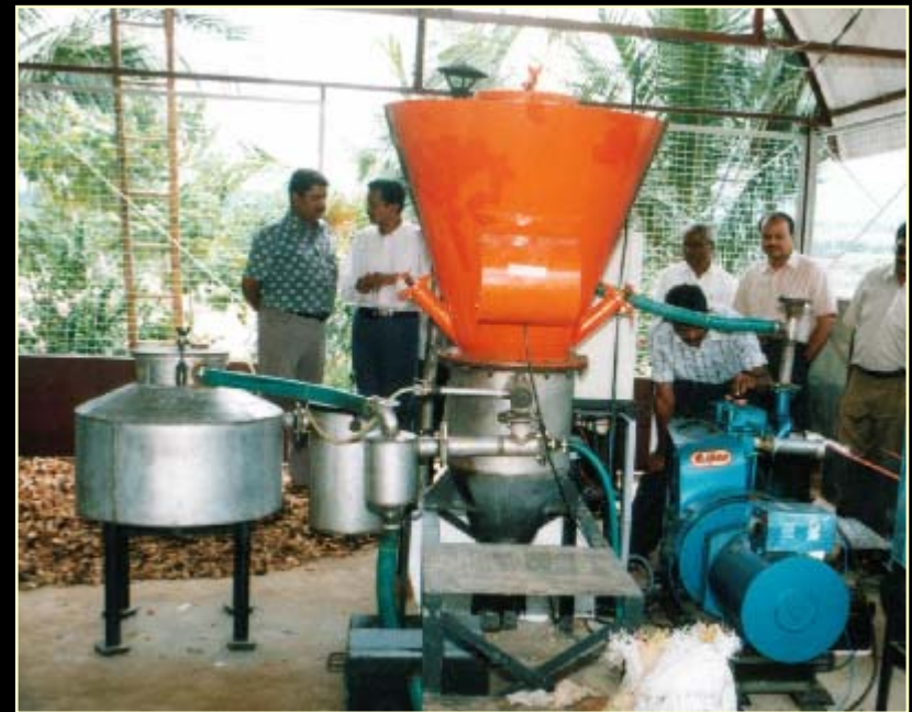
Gasifier Model: 1 X GAS-9 Odanduthurai, Coimbatore
