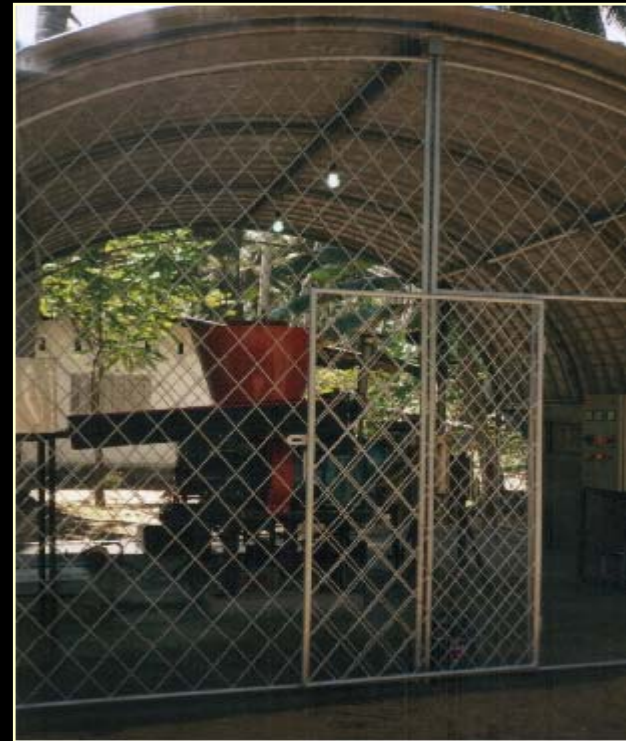
Gasifier Model: GAS-4
