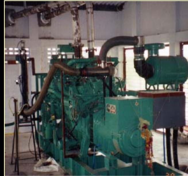
System Package : GAS-200
