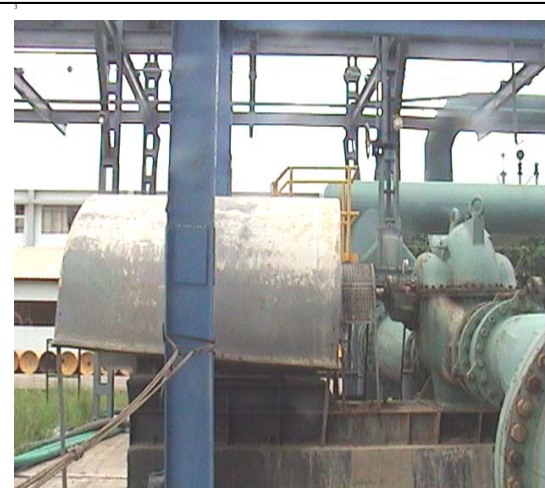
HP Cooling Water PP
