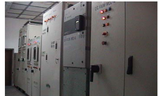
VFD Panels installed in CCU
