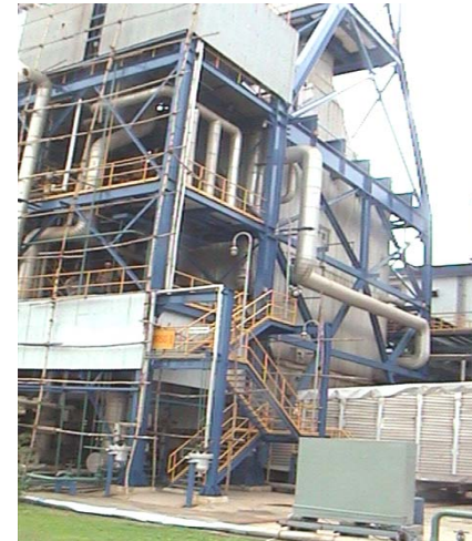
HEAT RECOVERY STEAM GEN. - 1
