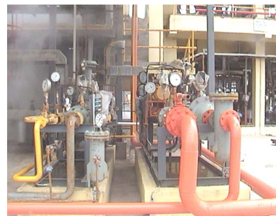
Hydrogen Control Station
