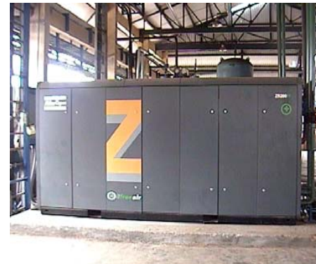
Atlas make Air Compressor
